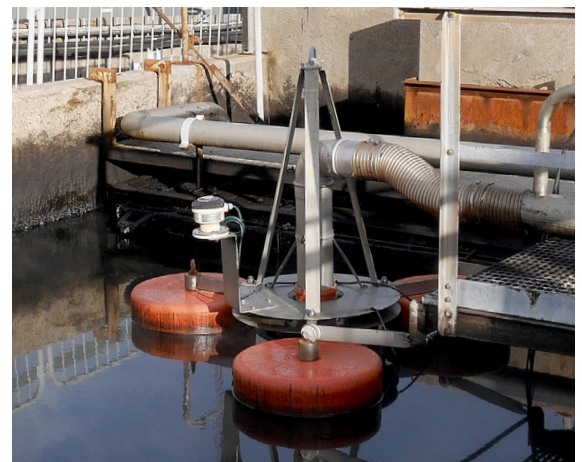
An Ultra-SurfCleaner operating in an API separator.
